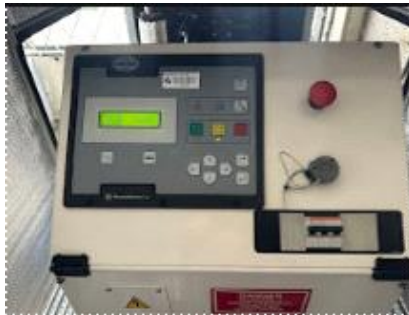
PANEL DE CONTROL
